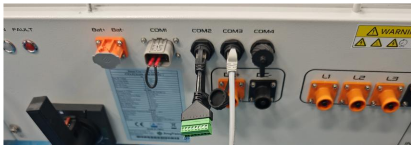
Fig5.3 CAN Bus Network Port Connection
